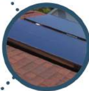
SOLAR HOT WATER
